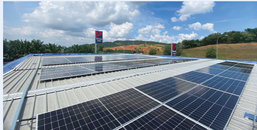
Our retail service stations are equipped with solar power panels supplying renewable energy
