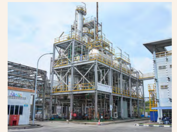
We completed our 30% plant capacity expansion at our Lumut POME Plant in February 2022.
