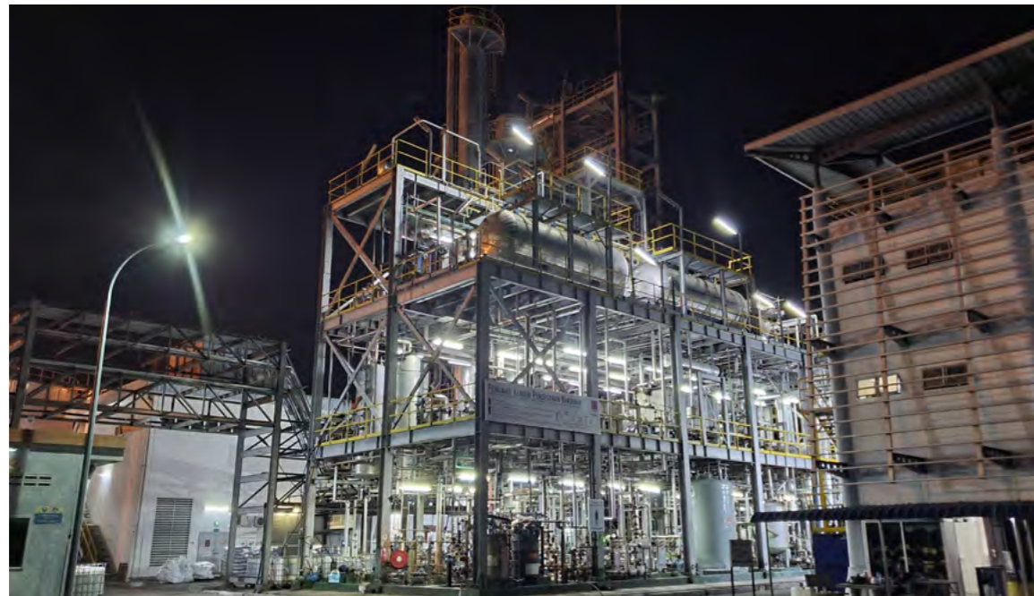
LED lighting installed at Lumut POME Plant
