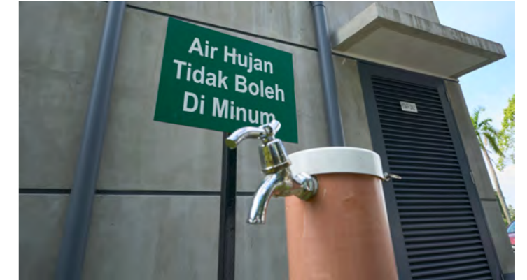
We installed rainwater harvesting system to collect and store rainwater for basic cleaning at Petron service station
