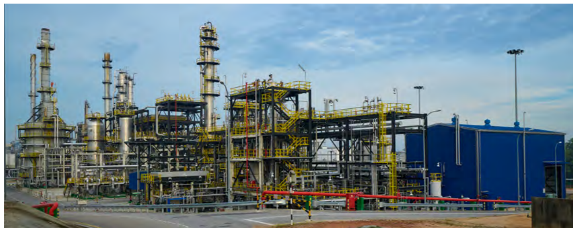
The BSR unit (in blue) was designed to recover sulphur from the DHT (in yellow trimming).
